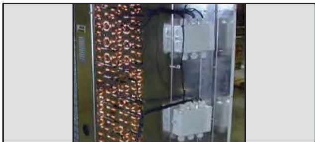
High grade electrical panel for fan motors and heaters, indicating clearly the electrical connections.
